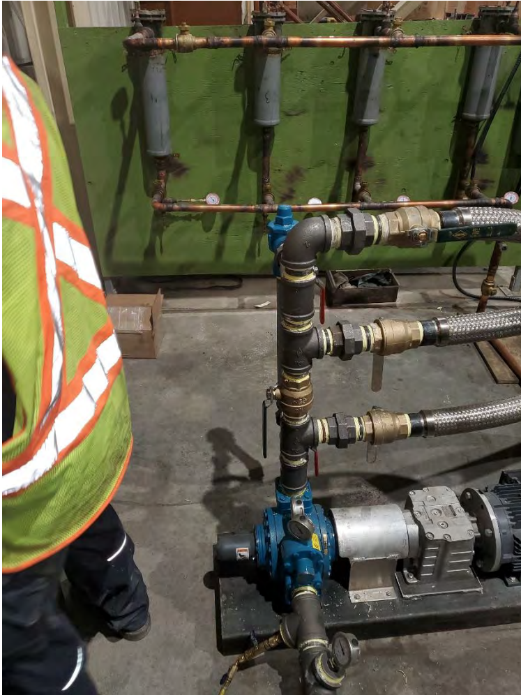
Figure 6 Pompe de recirculation
